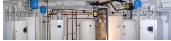
Figure 5: wide view of the technical room equipment
