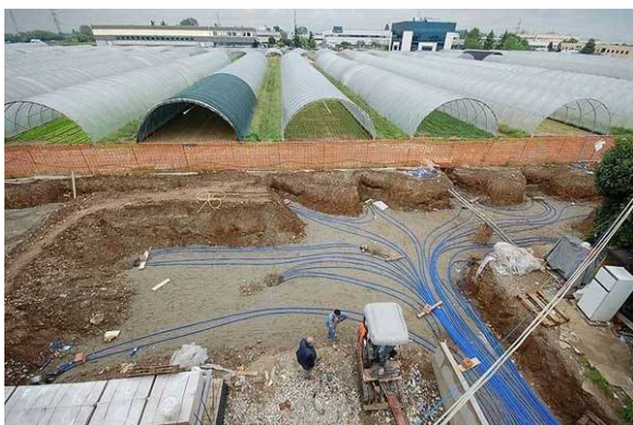
Figure 3: one of the three closed boreholes fields (F1 building): the 4 th from the left is the incorrect depth borehole n.47
