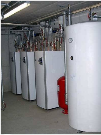
Figure 2: One of the three technical rooms; you can see heat pumps and 750l buffer tank
