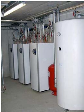
Figure 2: One of the three technical rooms; you can see heat pumps and 750l buffer tank
